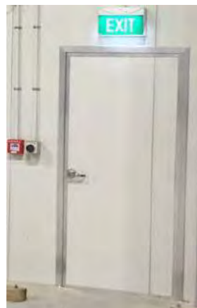
Coldstore PA Door
