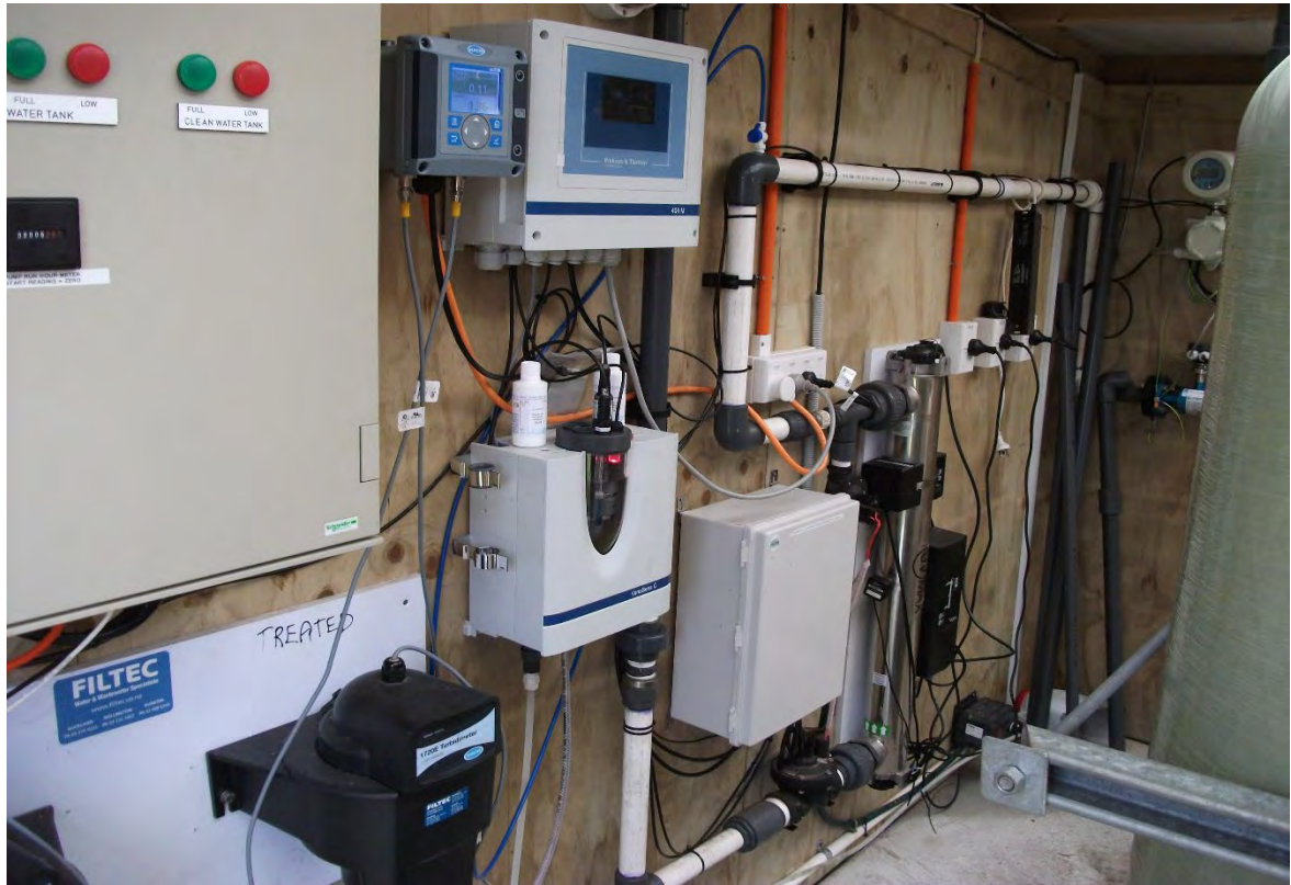
Kaingaroa Water Treatment Plant
