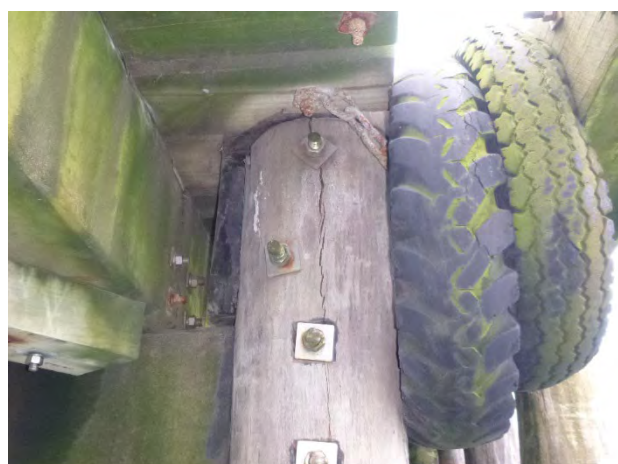
Figure 3-5: Owenga damage to bollard pile
