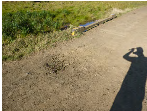
Figure 4-18: Thistle Clear (#P4) approach potholes
