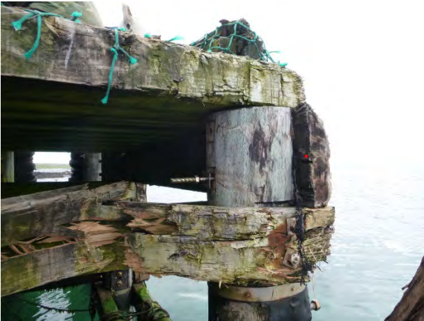
Figure 3-6: Owenga launch platform damage
