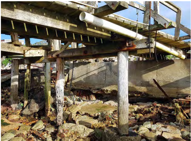
Figure 3-16: Kaingaroa poor condition piles
