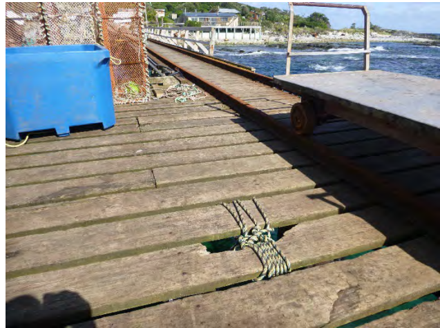
Figure 3-27: Kaingaroa damaged decking (2023)
