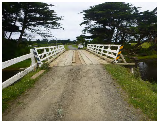
Figure 4-8: Maipito (#5) loose running boards
