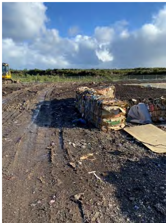
Figure 2-2 Owenga Landfill July 2023.
