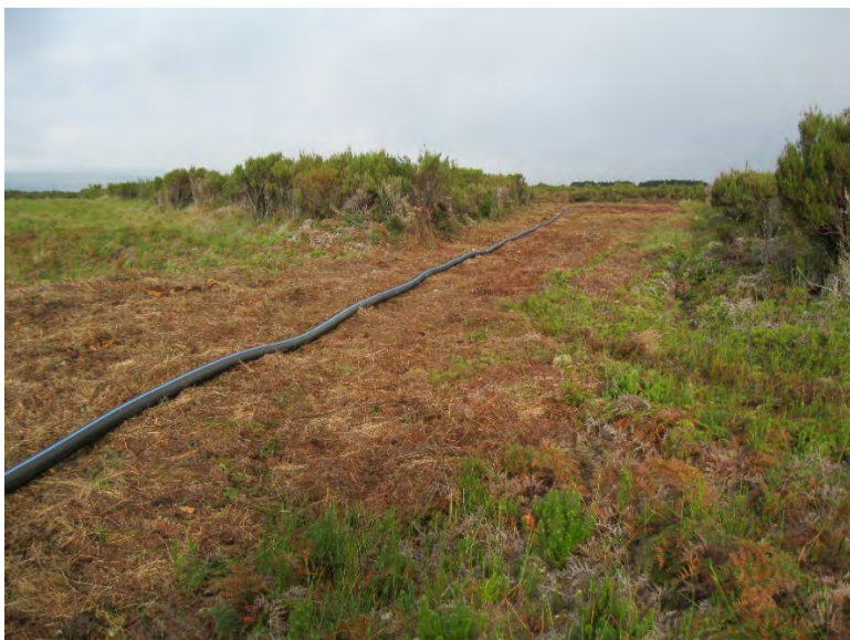
Figure 3-4: Top of the application area. The perforated pipe needs to be made as level as possible.
