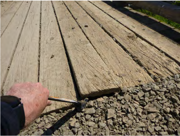
Figure 4-9: Awamata (#10) loose running boards
