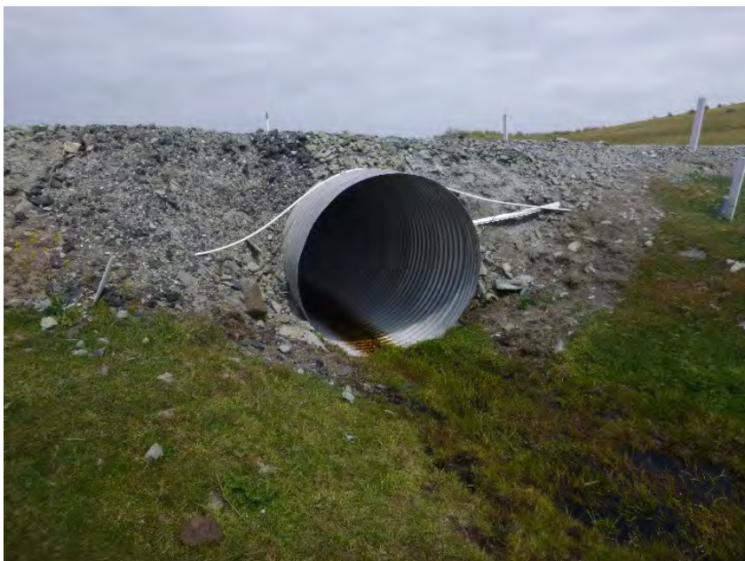
Figure 3-3: Waikawa (#23) cover issues upstream view
