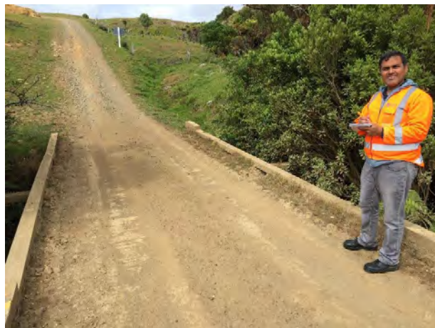
Figure 4-2: Typical dirt/gravel build-up on standard plank decking
