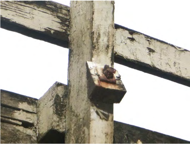
Figure 4-19: Lower Nairn (#20) rusted kerb bolts
