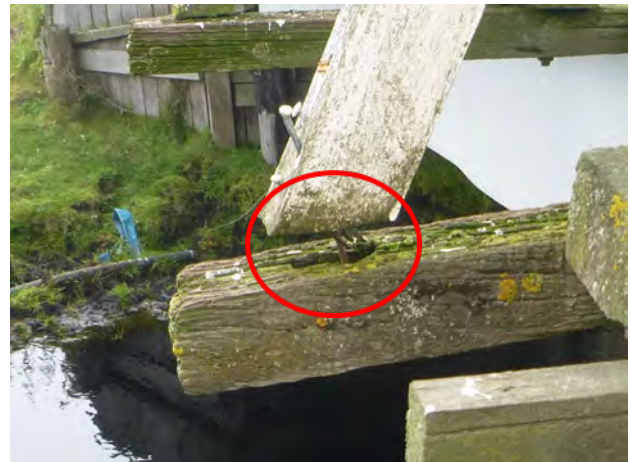
Figure 4-20: Washout Creek (#3) inadequate fixings
