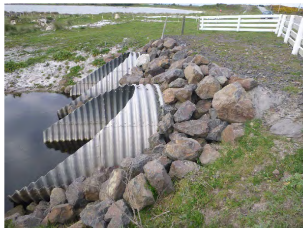
Figure 4-14: Waikato (#8) rock placed too steep
