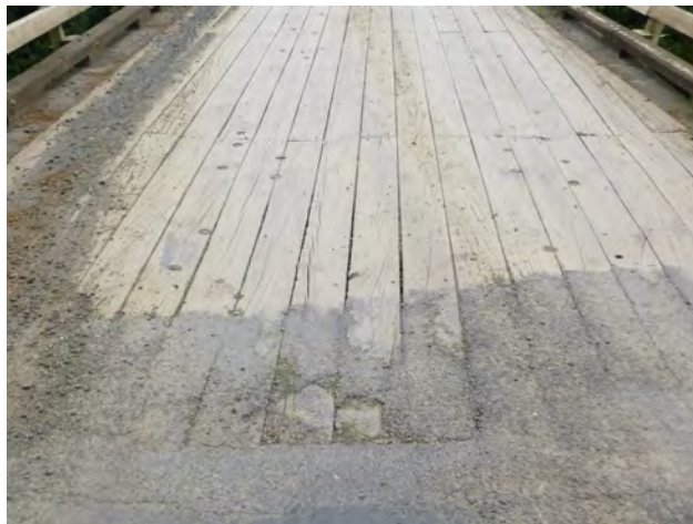
Figure 3-31: Te Awainanga deck wear
