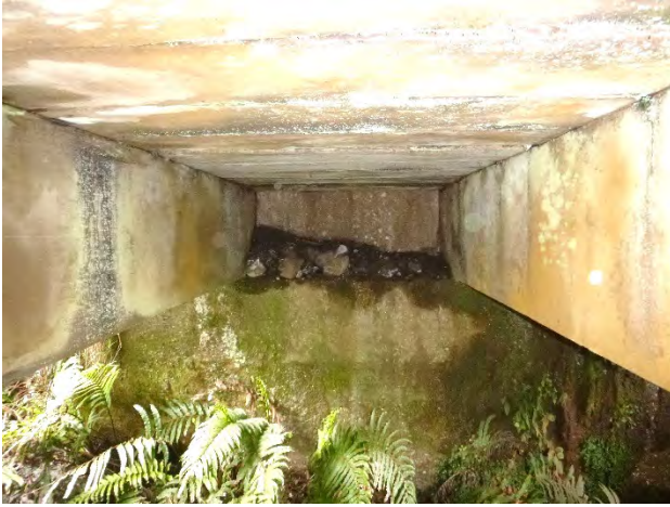
Figure 4-5: Kiringe (#12) debris on bearing shelf
