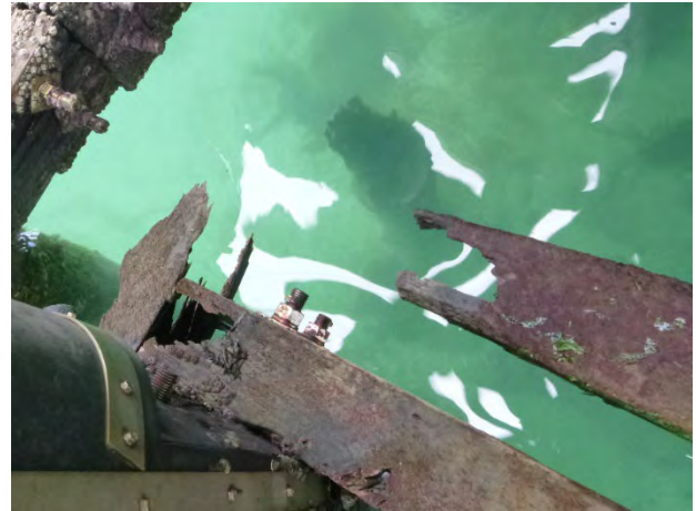
Figure 3-7: Owenga Toredos worm damage
