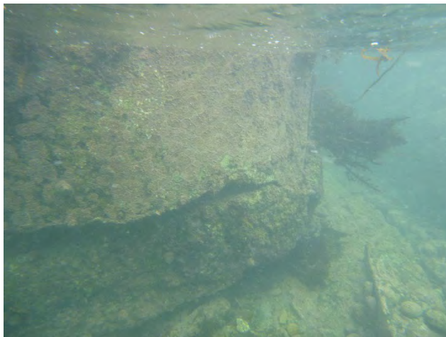
Figure 3-25: Kaingaroa undermined founding
