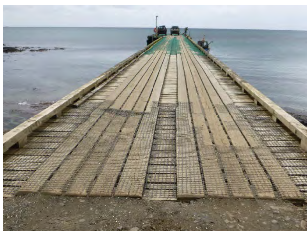
Figure 3-4: Owenga skid cladding failing
