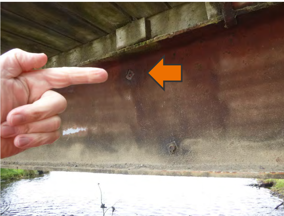
Figure 4-21: Maipito Bridge broken cross brace rod
