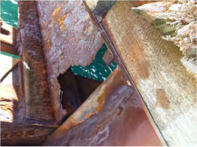
Figure 3-22: Kaingaroa heavy section loss
