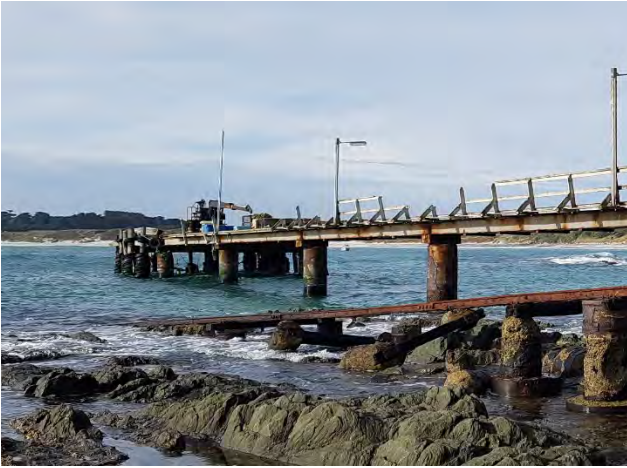
Figure 3-20: Kaingaroa damaged handrail
