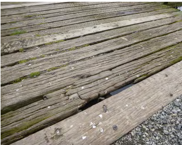
Figure 4-7: Washout Creek (#3) broken and loose deck planks
