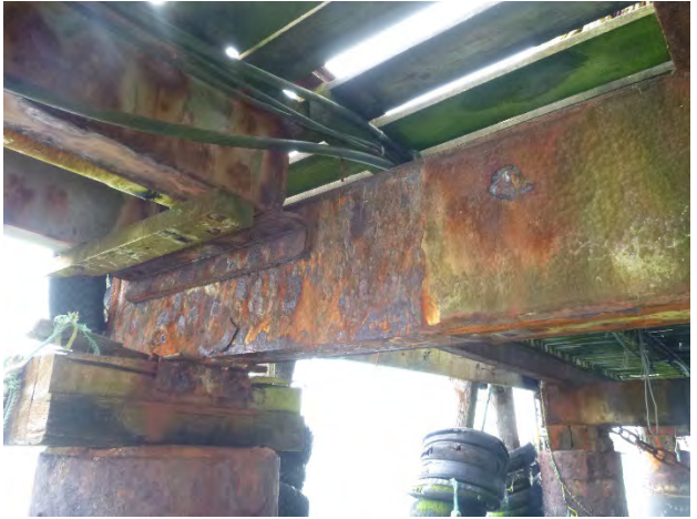
Figure 3-23: Kaingaroa heavy section loss
