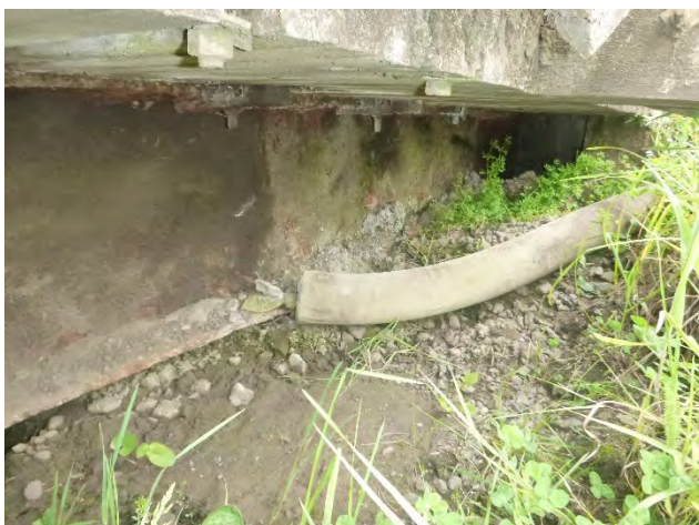
Figure 3-30: Te Awainanga debris on TR abutment
