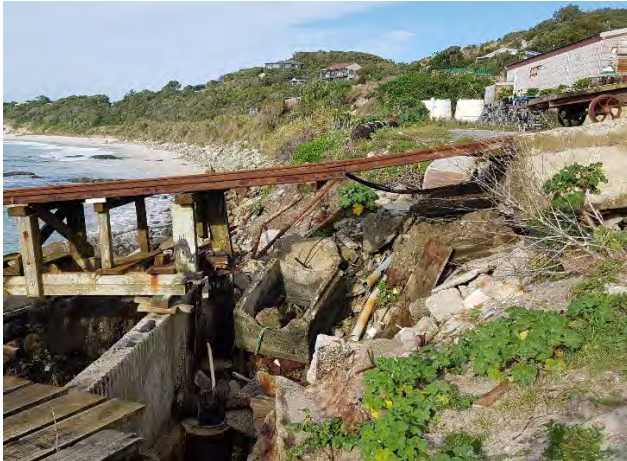
Figure 3-14: Kaingaroa poor ramp support
